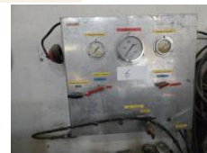
Lot.6 Tableau air distribution air + 2 consignes BSO
